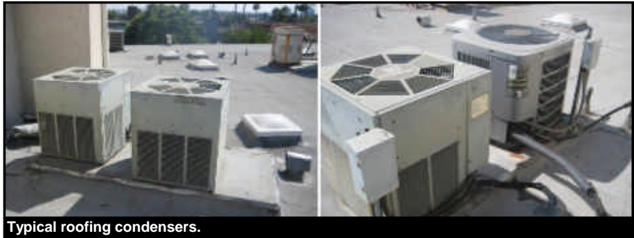
Typical roofing condensers.
