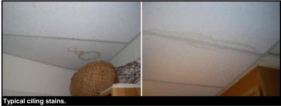
Typical ceiling stains.
