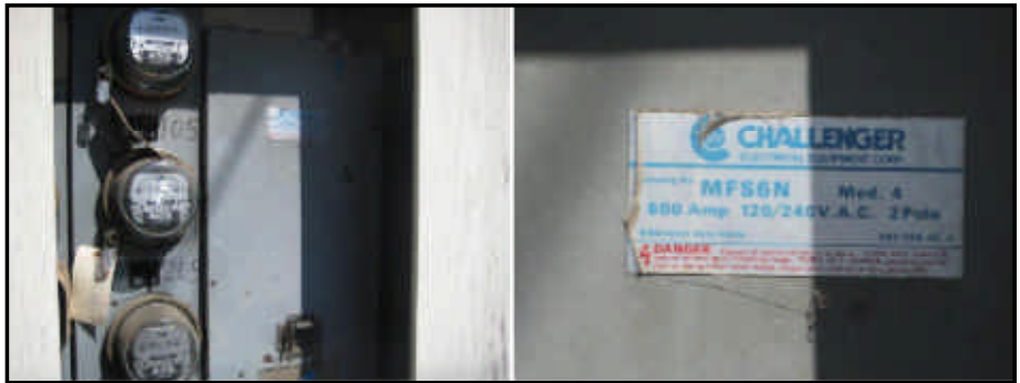
The main electrical panel is located on the rear exterior wall of the building.
