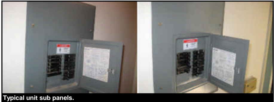
Typical unit sub panels.
