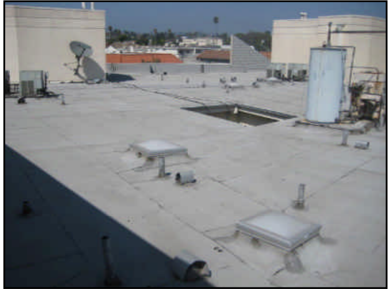
The roofing material on the low sloped roof is rolled composition roofing.
