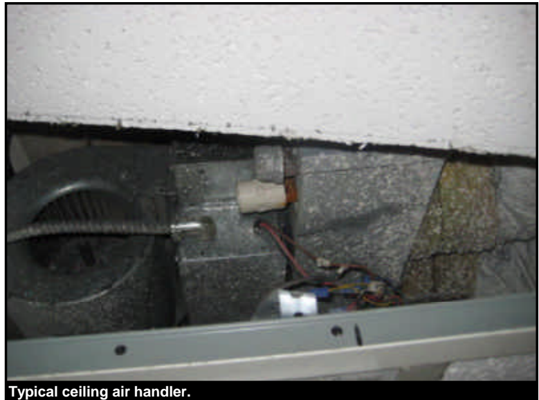
Typical ceiling air handler.
