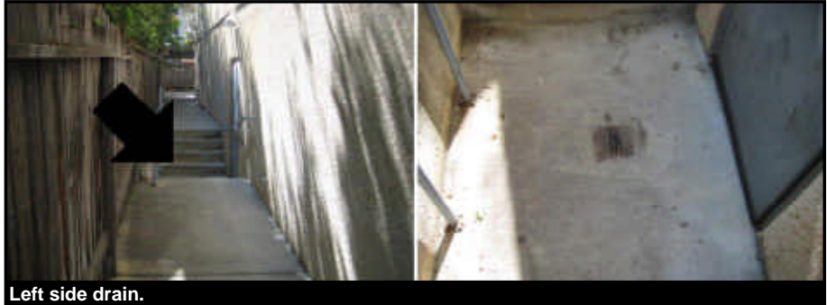
Left side drain.
