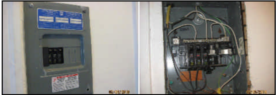
Typical sub panel.
