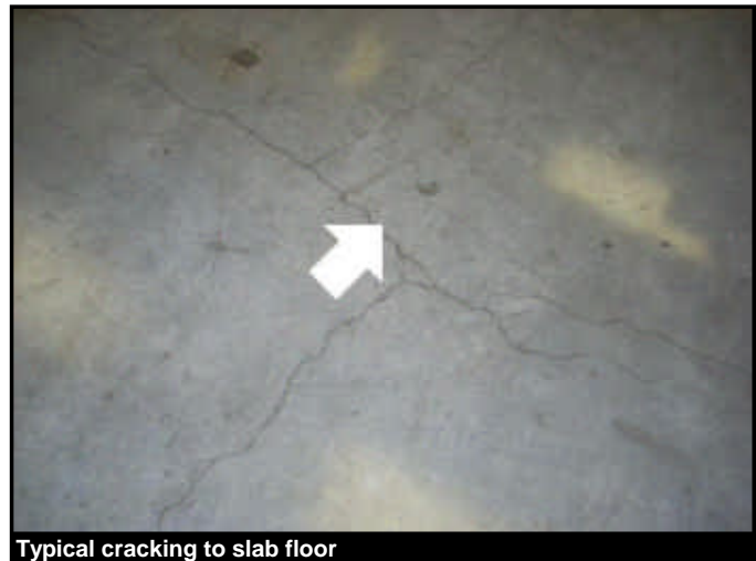
Typical cracking to slab floor
