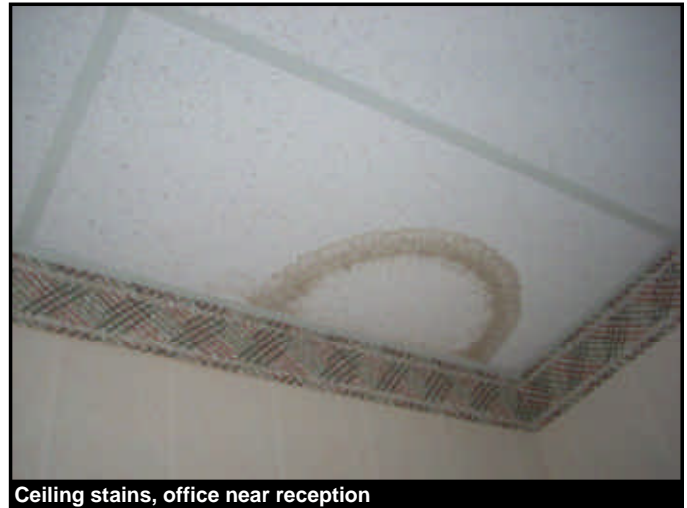
Ceiling stains, office near reception
