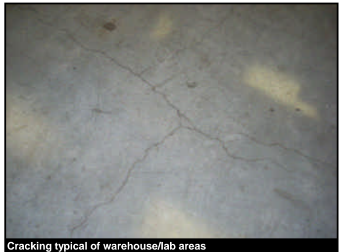
Cracking typical of warehouse/lab areas
