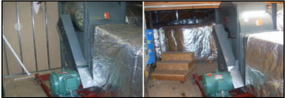
High volume fans appeared serviceable
