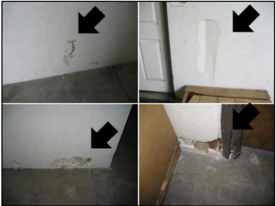
Pictures of the wall damage in the warehouse area.
