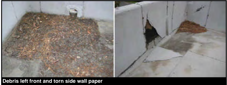
Debris left front and torn side wall paper
