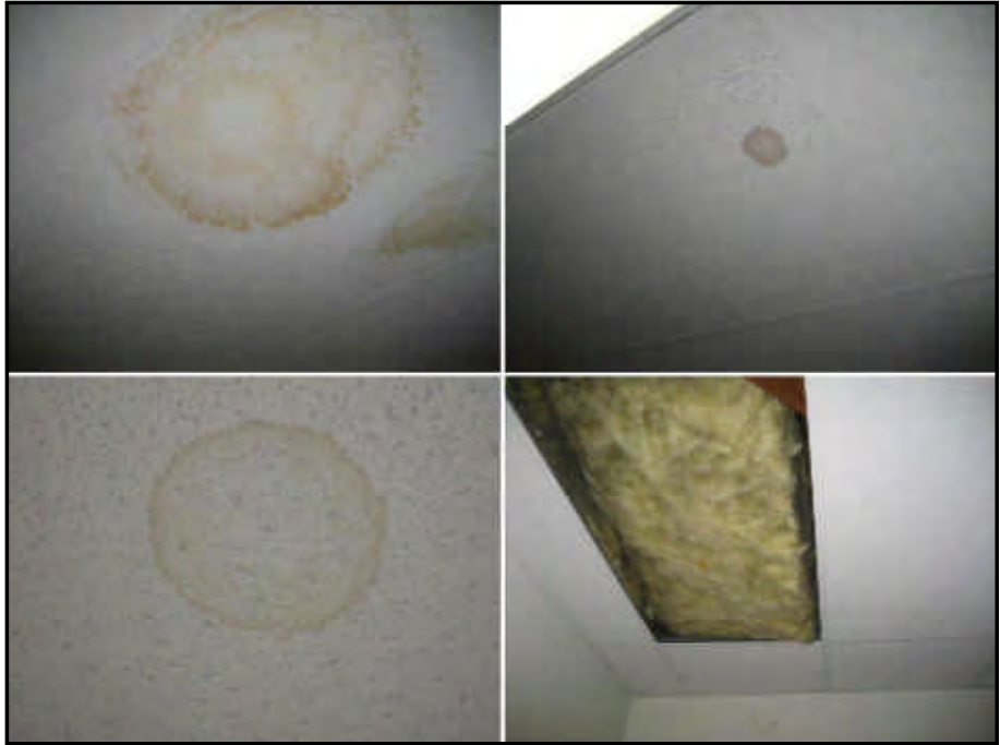
Picture of the moisture stains and damage to the ceiling.
