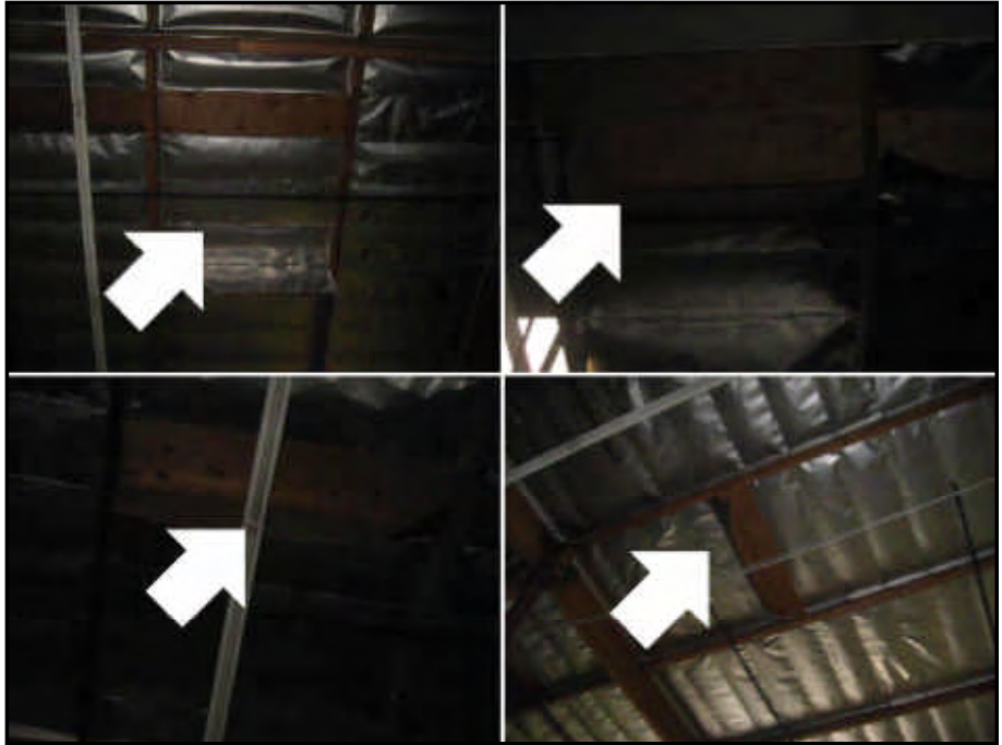
Pictures of the ceiling insulation falling down from the ceiling.
