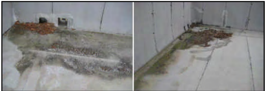
Debris around drains.
