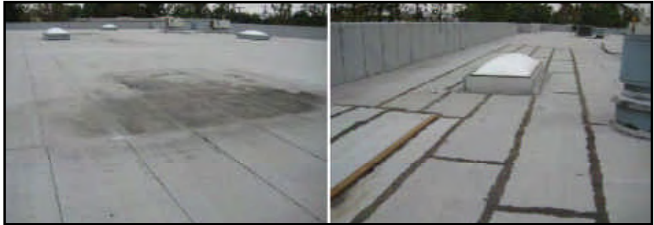
Flat area left and patched area right
