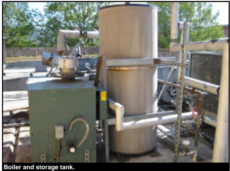
Boiler and storage tank.
