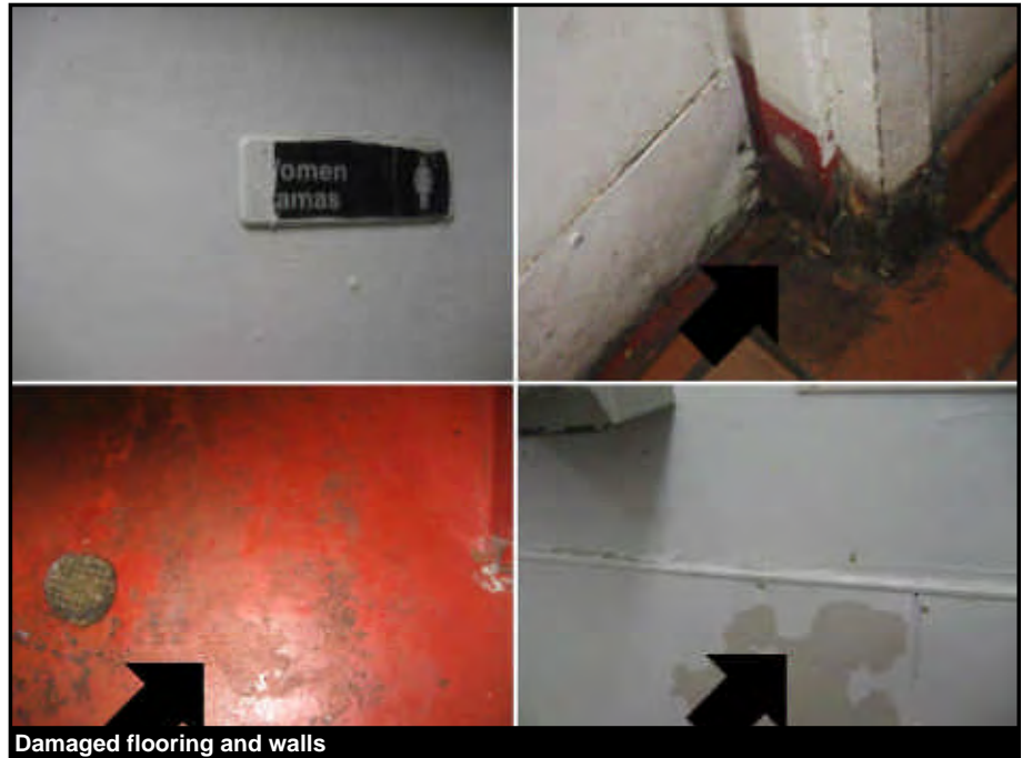
Damaged flooring and walls
