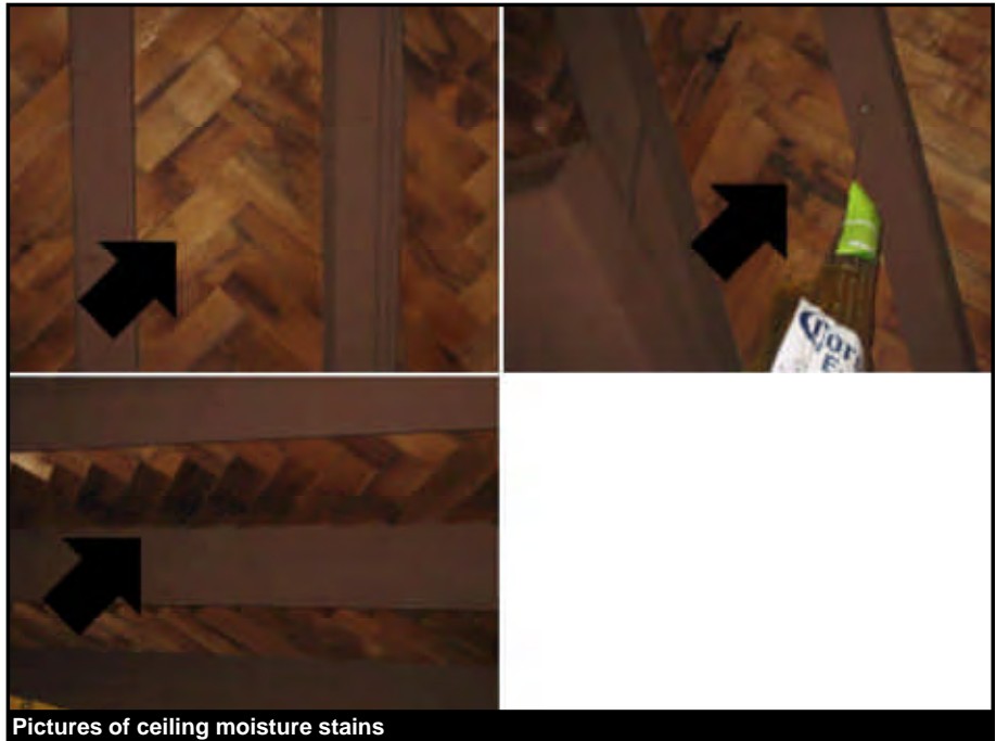
Pictures of ceiling moisture stains Needs Attention:
