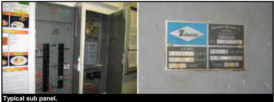
Typical sub panel.
