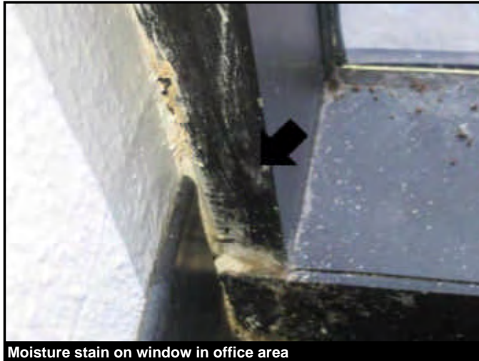
Moisture stain on window in office area
