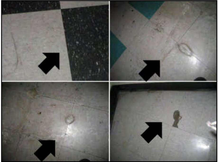
Pictures of the worn and damaged floors.
