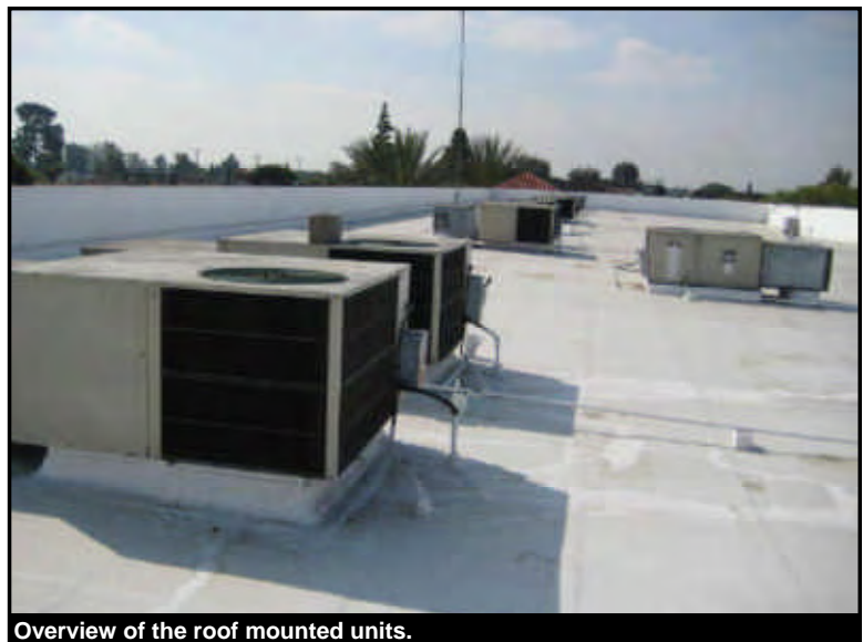
Overview of the roof mounted units.
