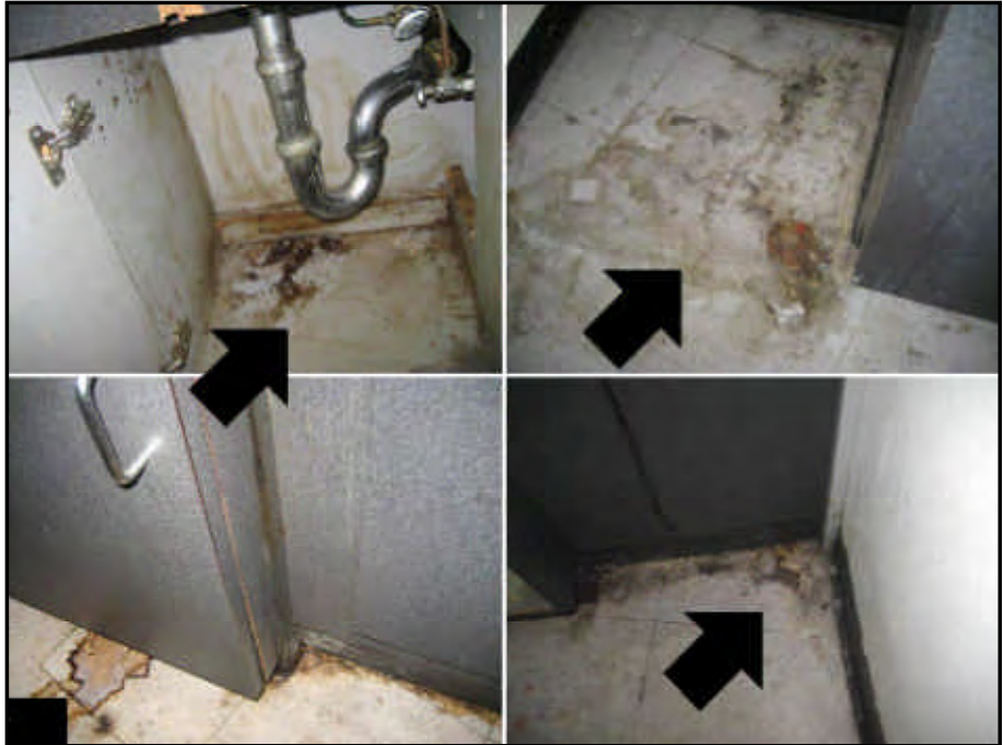
Pictures of the moisture stains on the flooring.
