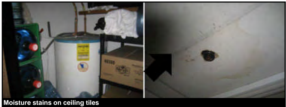
Moisture stains on ceiling tiles Mop closet
