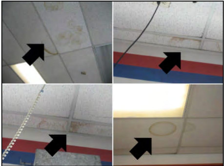
Pictures of the moisture stains on the ceiling.
