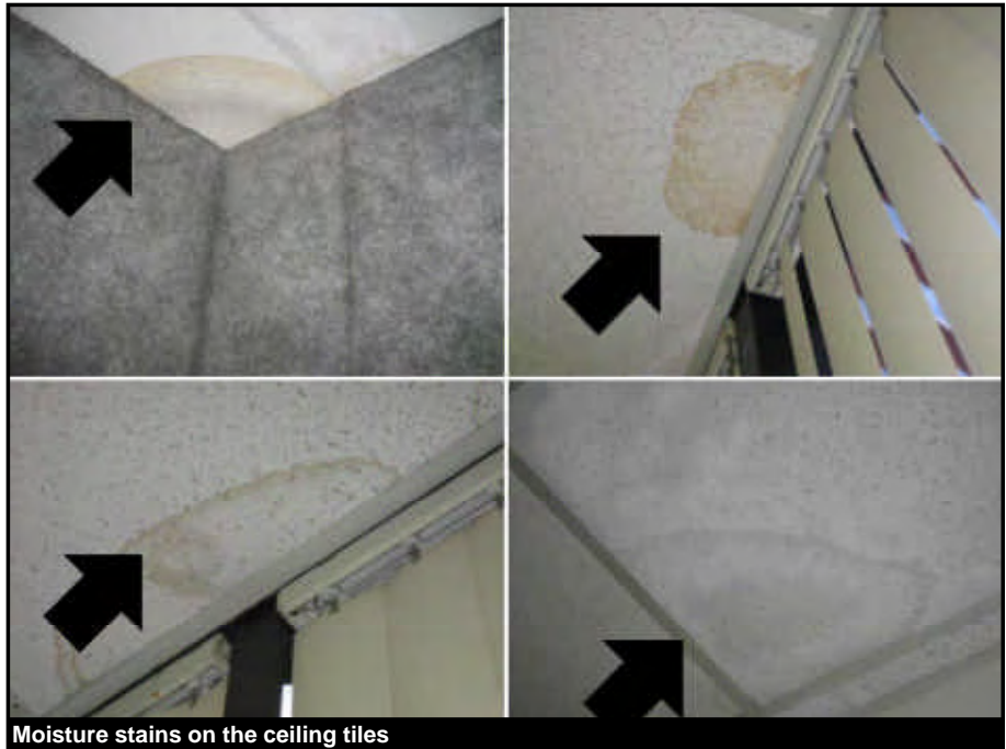
Moisture stains on the ceiling tiles
