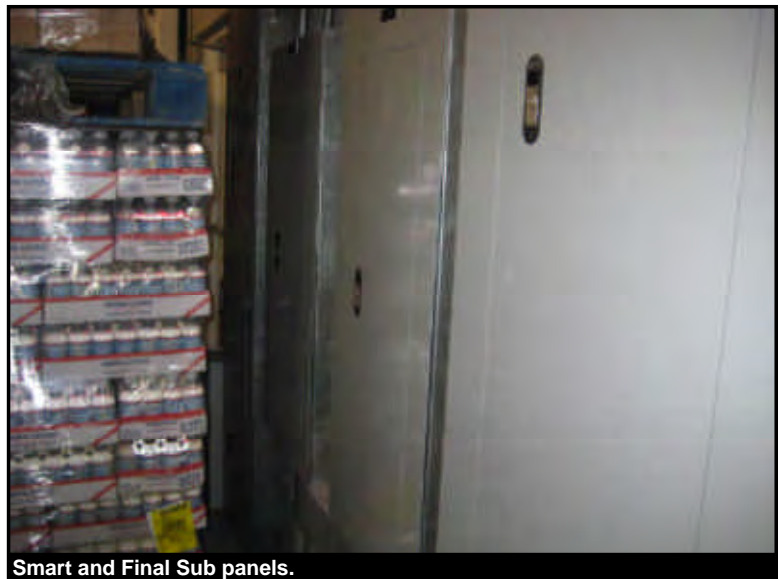
Smart and Final Sub panels.
