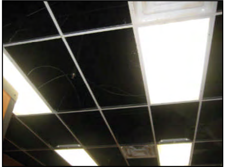
Serviceable - however there are ceiling tiles missing.
