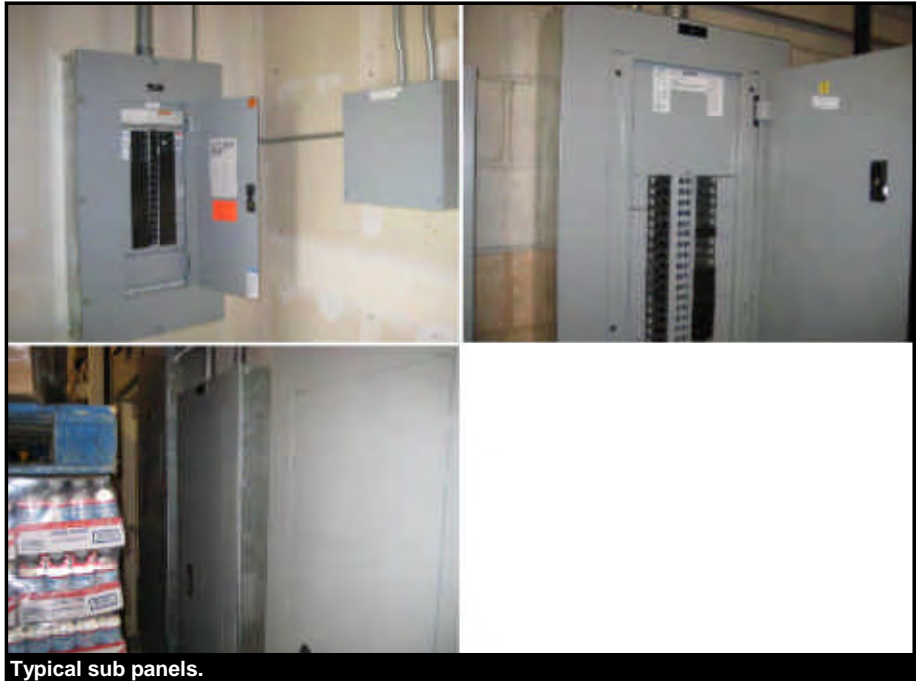
Typical sub panels.
